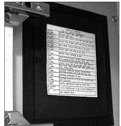
Fuse Panel Label located in bedroom.
