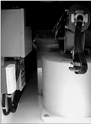
Power Cable Reel
